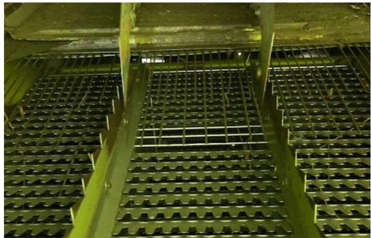
Photo 1 A fragment of a damaged sieve, made by welding the lamella to the axis of rotation.
